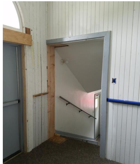
Pre-installation view of interior stairway location leading down from main Museum display level to ground-level entrance.
